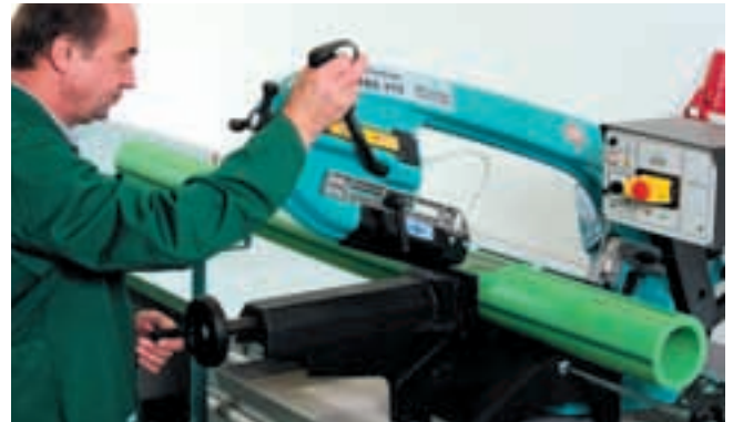
Before welding, the 160, 200 or 250 mm pipes are cut into the required lengths
