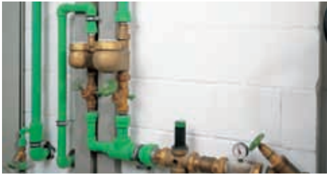
From the house connection station, cold water distribution, boiler connection and hot water distributor...
